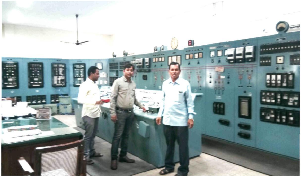
TBHES - DAM POWER HOUSE - CONTROL ROOM
